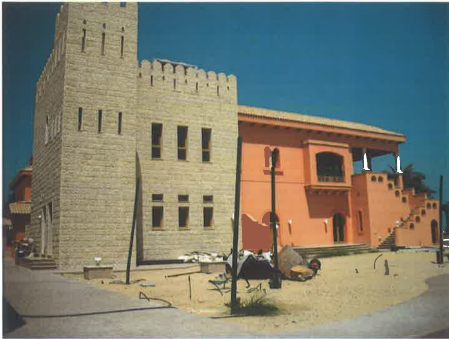
Decorative Grc Works for luxury Villa's at Palm Island (E-front Tip) Dubai.
